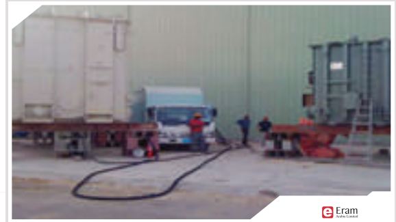
Mobile Oil Filtration Unit at Site
