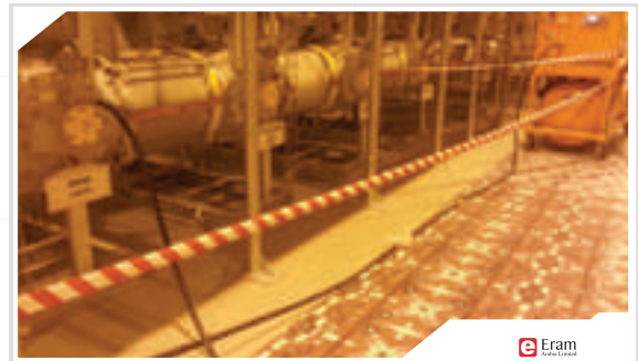
Dhahran Home ownership - 115KV S/S - 1A
