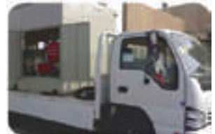
On Site Oil Filtration Services Filtration Machine with Capacity 6000 LPH
